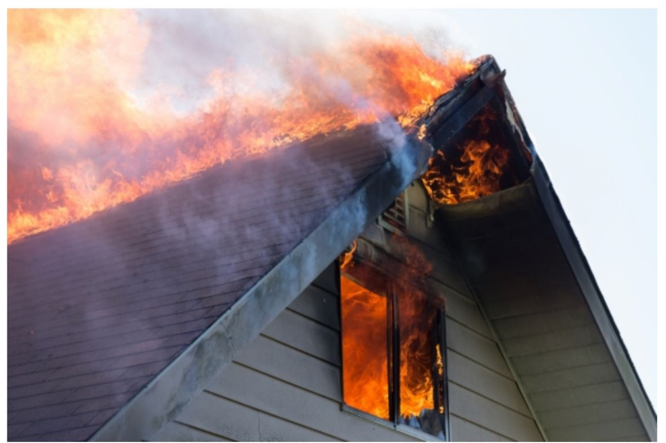
Embers can carry as far as a mile in the wind, and when they get into an attic, they can start a fire.
